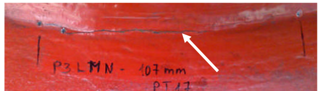
Intermediate equalizer beam crack (lower photo) that is obstructed by the pin ear plate in the upper photo.
